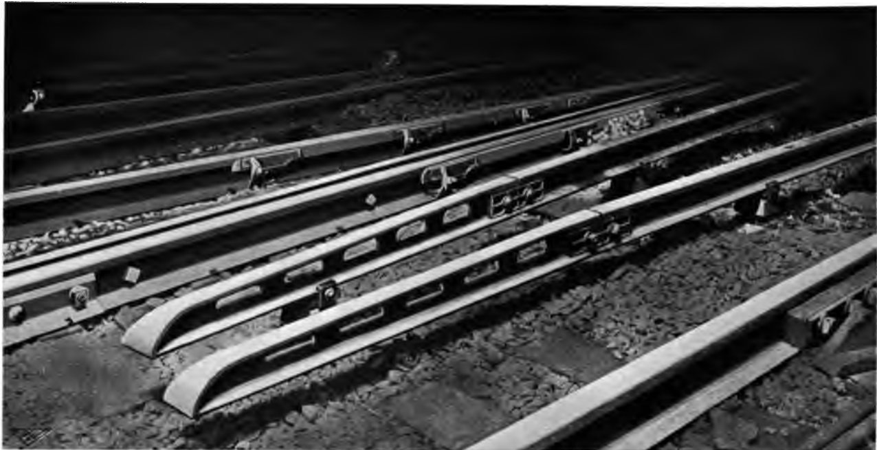
CONTACT RAILS, SHOWING END INCLINES
